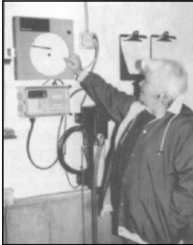
Maggie Becker, Dover city council member, checks the flow rate of the city’s new water treatment system.
